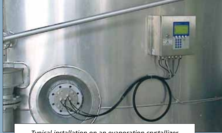
Typical installation on an evaporation crystallizer
