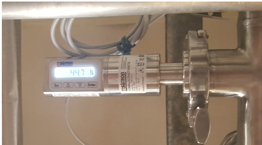
Cream line sensor installation
